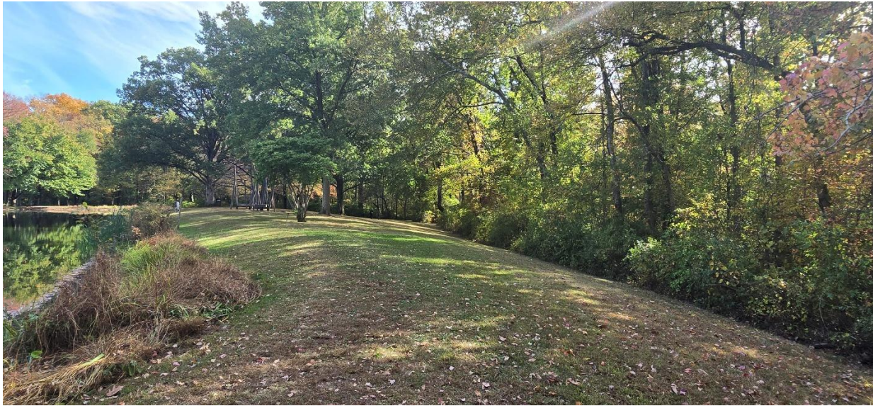
Figure 3. Earthen embankment (dam) of the IAS pond, showing crest and downstream slope (photo by the author, October 18, 2025).
